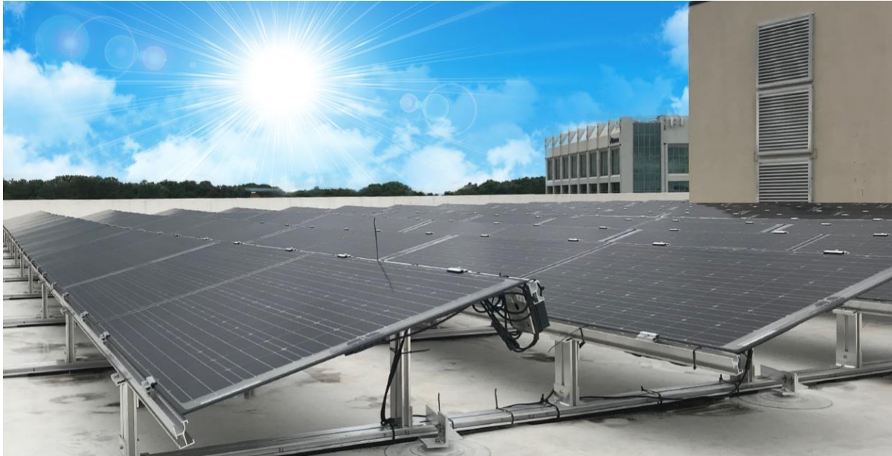
Solar panels on the first C-PACE solar project by Recurrent
